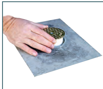
Apply primer and glue to the inside pipe fit cleanout and inside of the pipe. Insert the cleanout.
